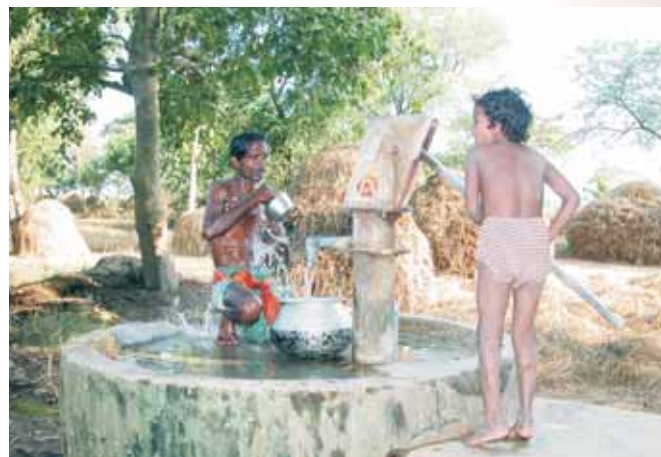
Hand pump installed as part of NALCO's CSR activities
