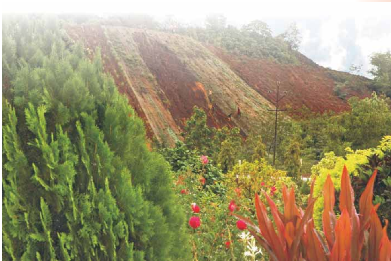
Dump slope stabilization with coir netting & lemon grass plantation at Sukinda Chromite Mine
